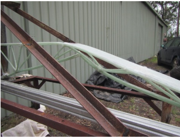
Crack bang and the load drops to the ground
